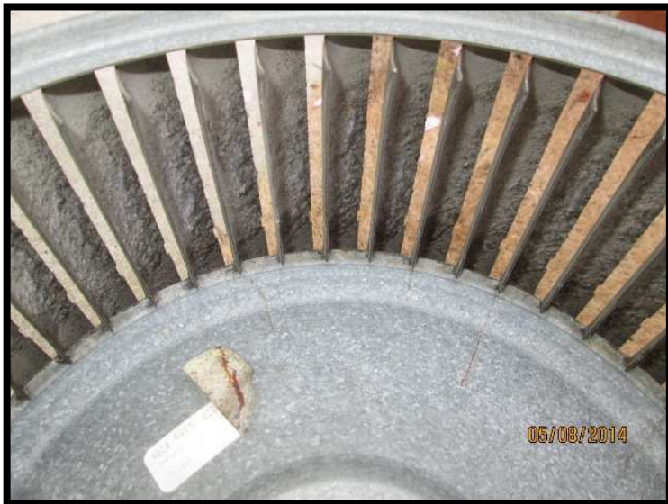
Blower wheel before
