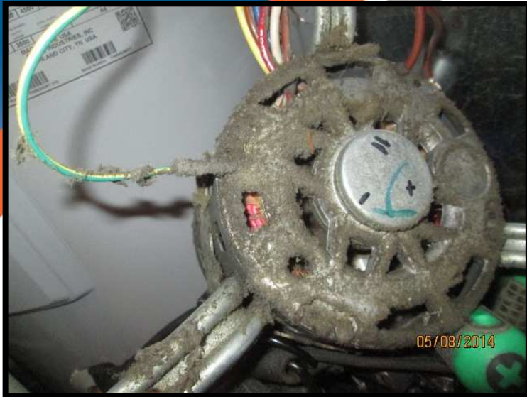
Blower motor before cleaning
