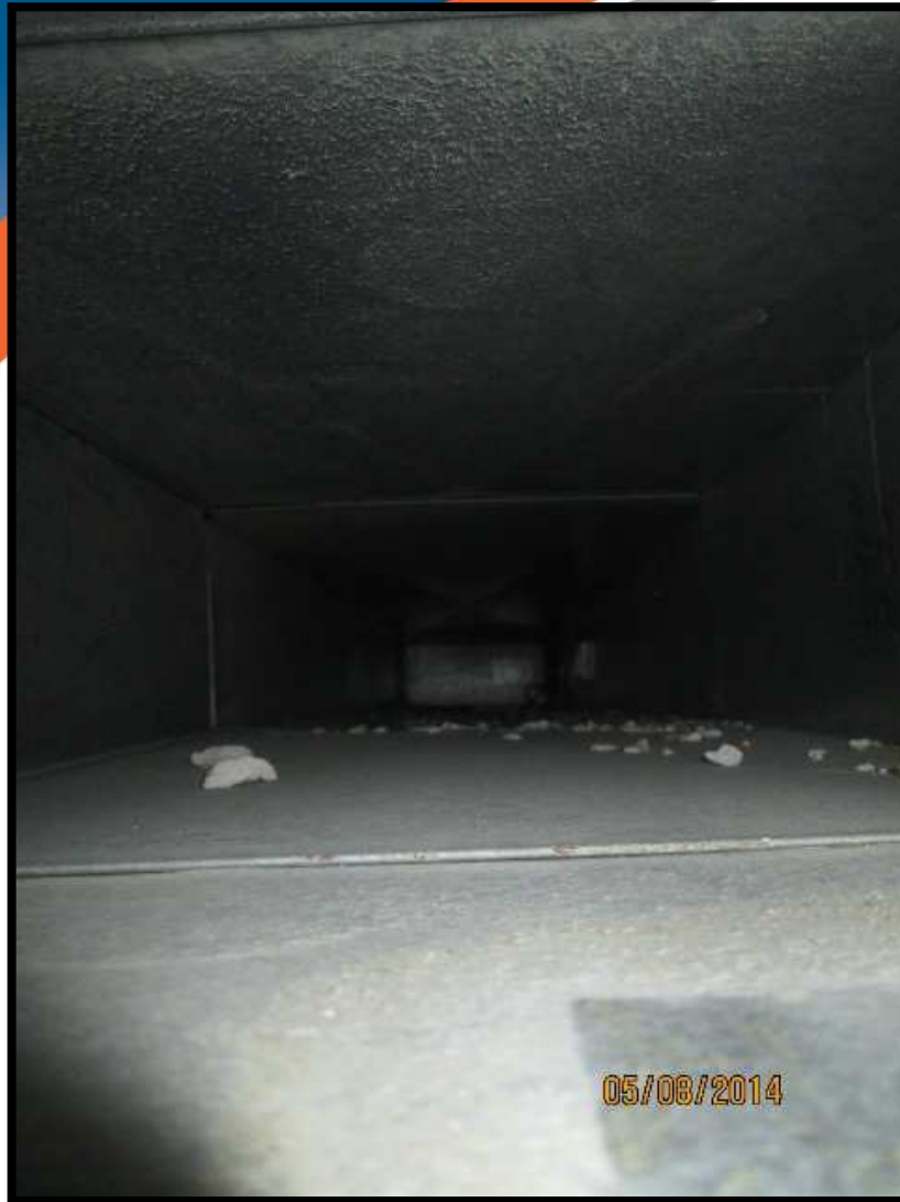
Supply trunk before cleaning
